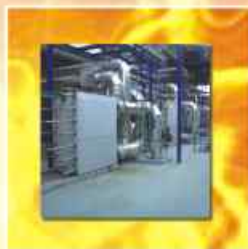
ASSEMBLY OF HEATING STATIONS
