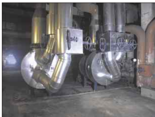
Installation of PSHE 9 exchangers as steam heaters (dismountable design, 2 x 16 MW output) at the Vresova plant, Sokolovska uhelna, a.s.
